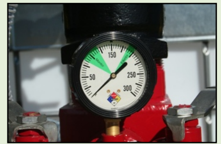
Appliance Ops. Gauges
